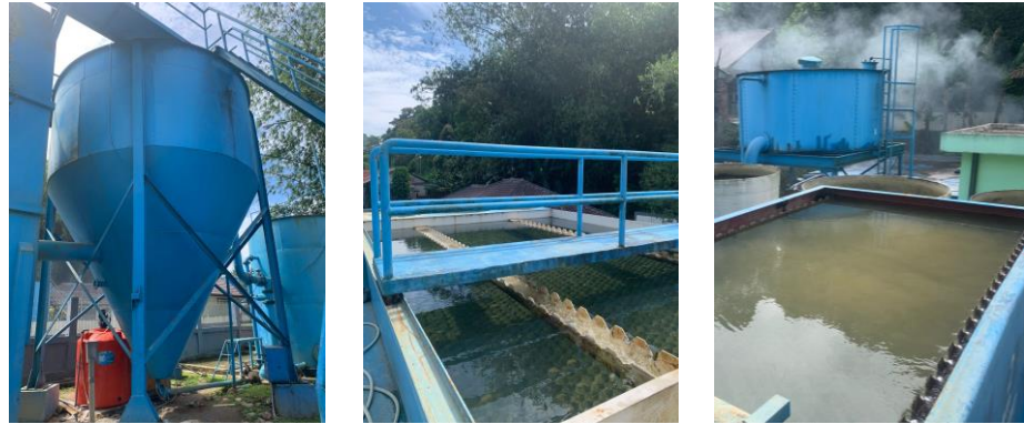
Gambar 5.5 Unit Sedimentasi (a). WTP Kerucut, (b). WTP Degreemont, (c). WTP Hexagonal.
